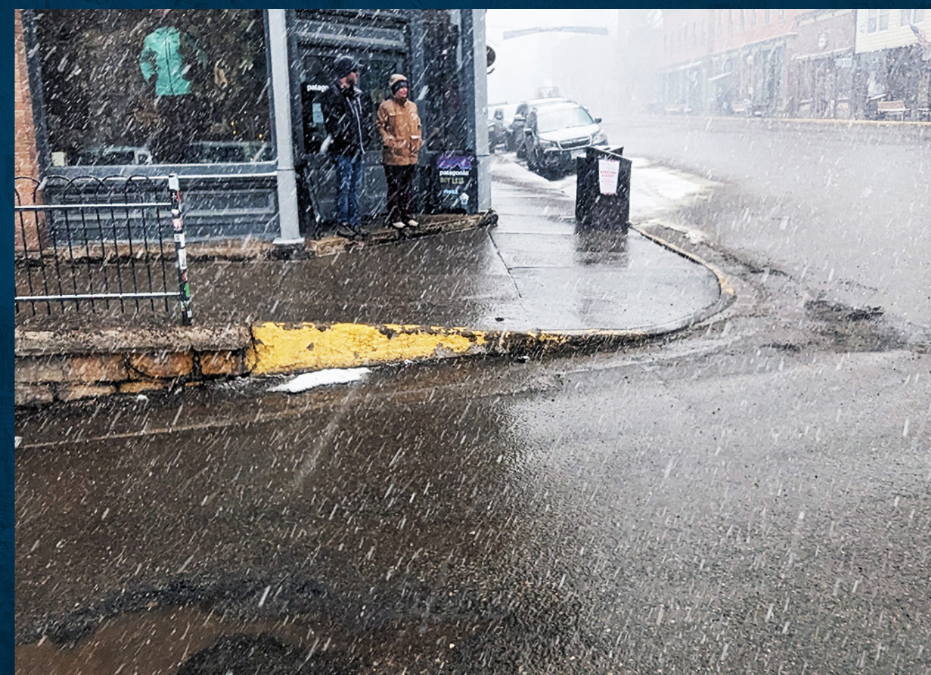
The intersection of Colorado Avenue and Fir Street featured aging pedestrian curb ramps that no longer met current accessibility standards.
