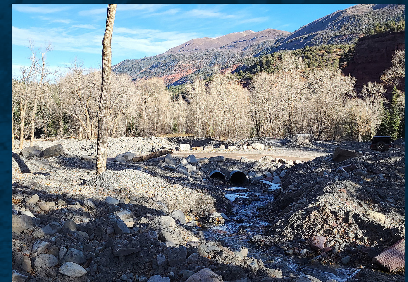
Two 48-inch culverts at the Corbett Creek crossing were unable to safely pass debris flows and typically required replacement after each event.
