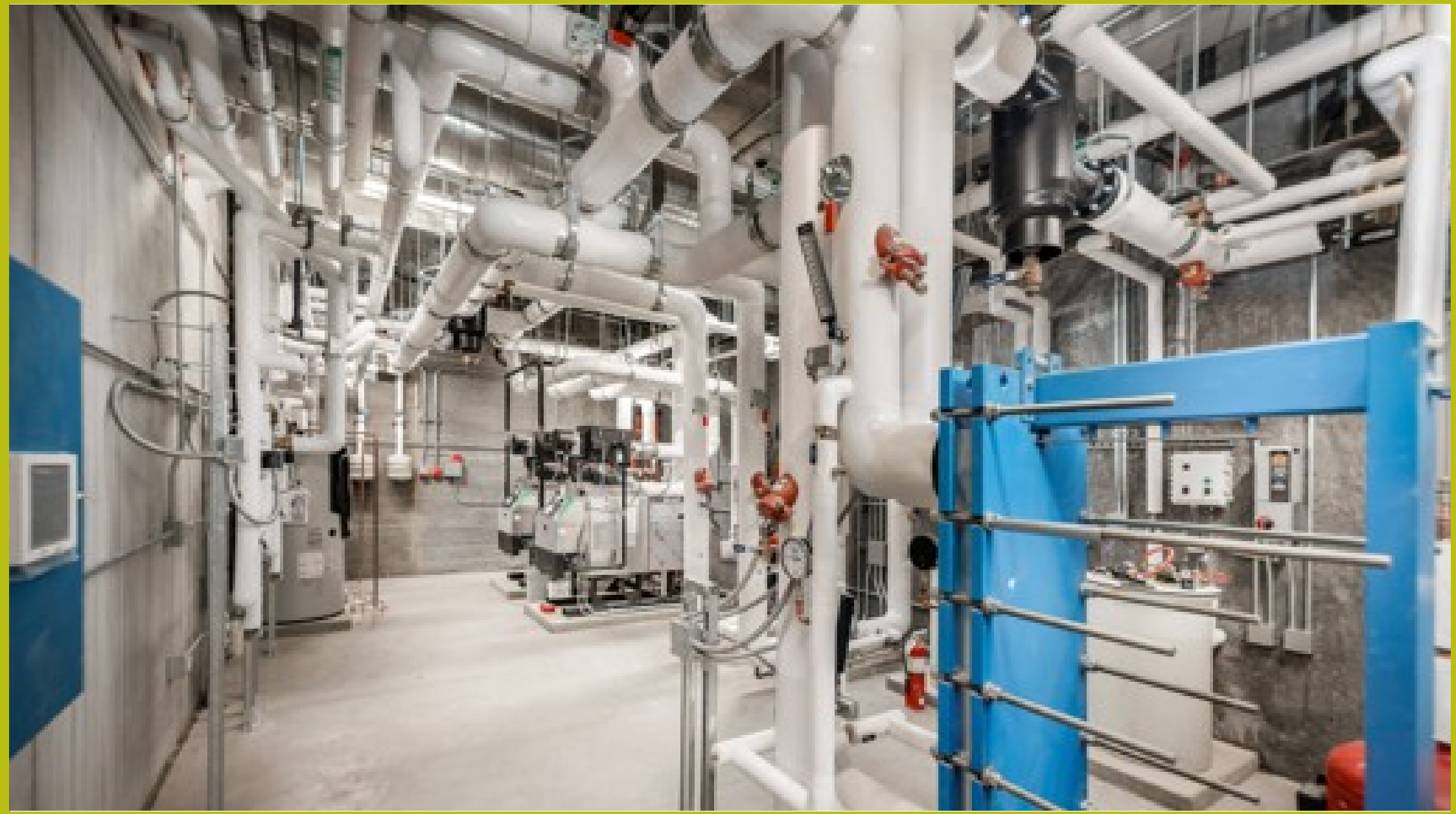
High-efficiency mechanical infrastructure supports the transit center's sustainability and operational goals.
